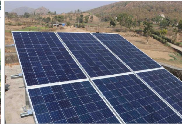
Solar power to facilitate water supply and electricity
