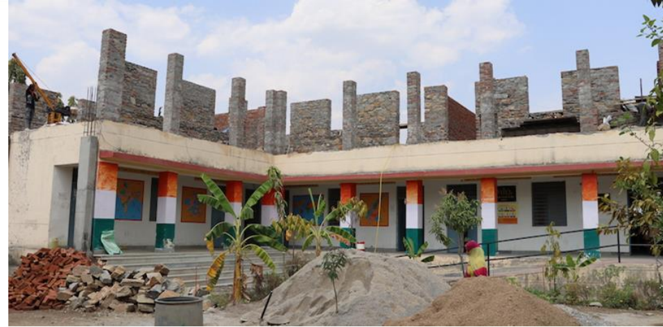
Science Laboratory under construction at Govt. Girls Sr. Sc. School at Khamnore
